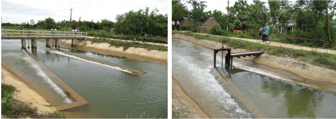
Photo 10.2. Vietnam: Phu Ninh Irrigation Scheme; Construction of Long Crested Weirs on the Main and Secondary Canals
