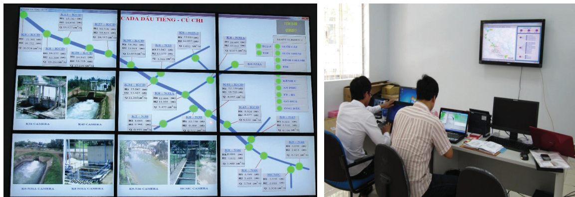
Photo 10.3. Vietnam: Dau Tieng East Main Canal; SCADA under Operation
