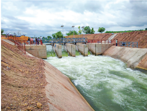
a. Automated Canal Gates
