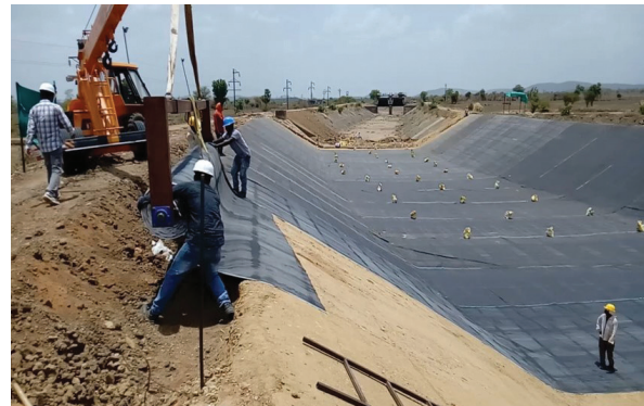
b. Maharashtra State, India: Lining of a Section of the Pench Main Canal with Bituminous Geomembrane
